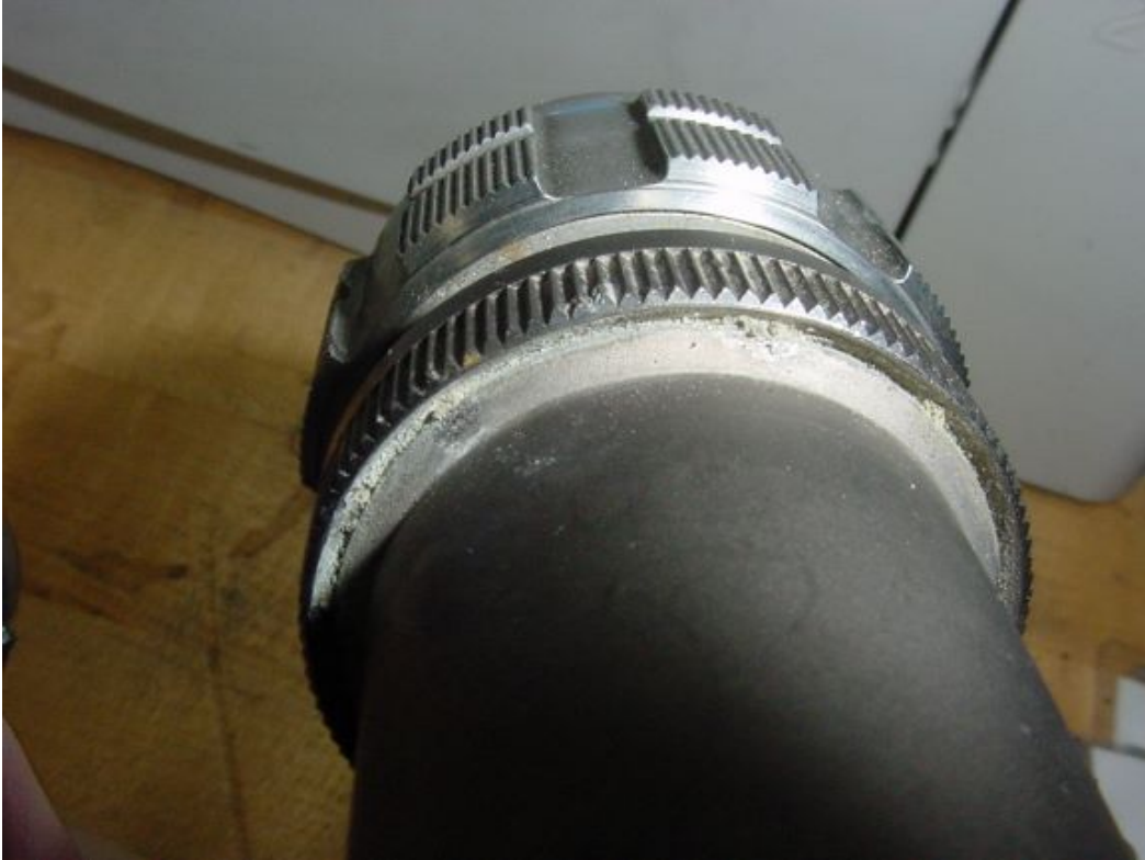
Engine control harness (corrosion on multiple backshells)
